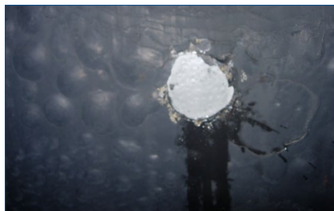
Blistering of coating with low cross-link density
