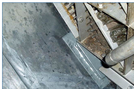
Inspection eight years later
